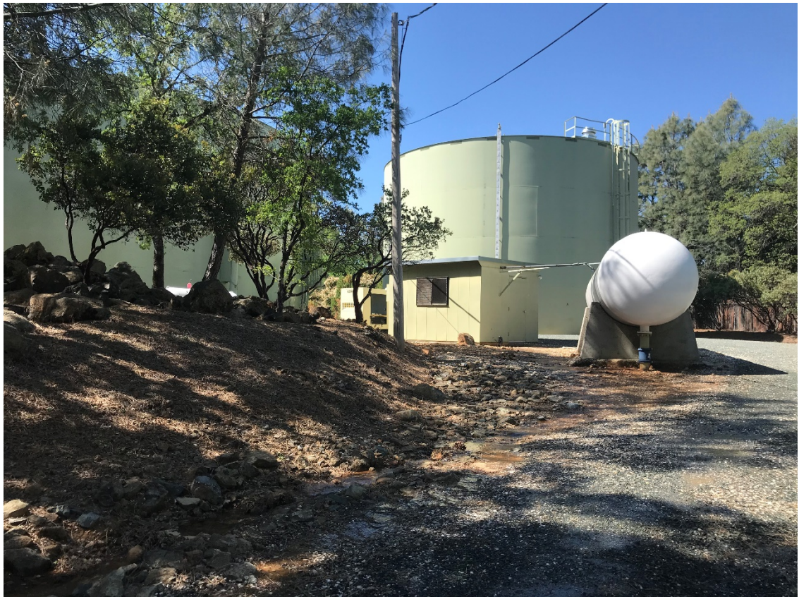
Existing pump station building, pressure tank, and storage tank from entrance, south view
