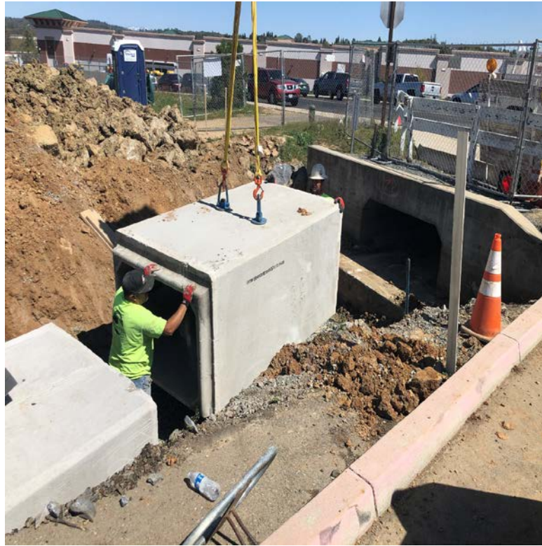
Developer Installed Project
